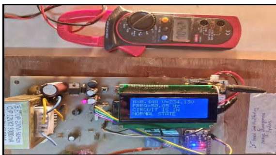
Fig. 12: Normal Circuit Condition while connected to a 100W Bulb
